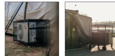
Split unit HVAC
